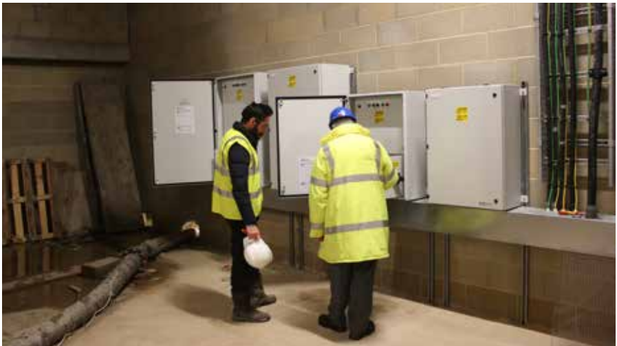
Typical Combination ATS units fully installed
